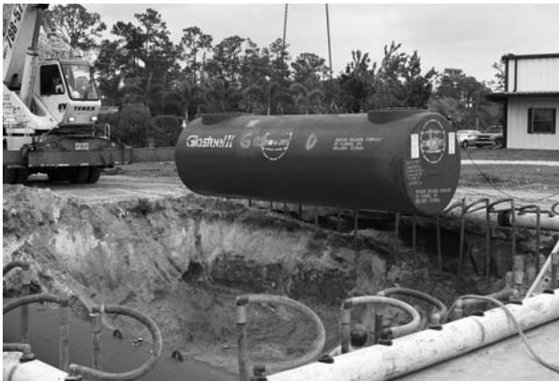
Fuel tanks at the District Office were replaced per EPA and Florida mandates
