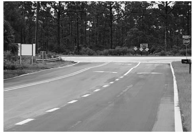
An asphalt overlay was recently applied to Haynie Lane in Jupiter Farms
